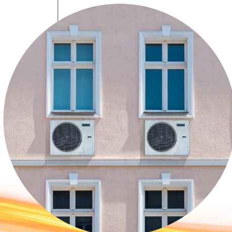
Facade with conventional outdoor units
